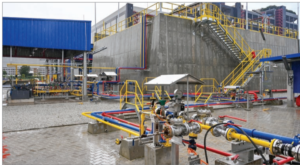
Being the first LPG bottling plant to be built in Singapore in about 40 years, the new bottling plant at 43 Jalan Buroh is equipped with enhanced safety features, such as the concrete bunker that holds its LPG tanks
